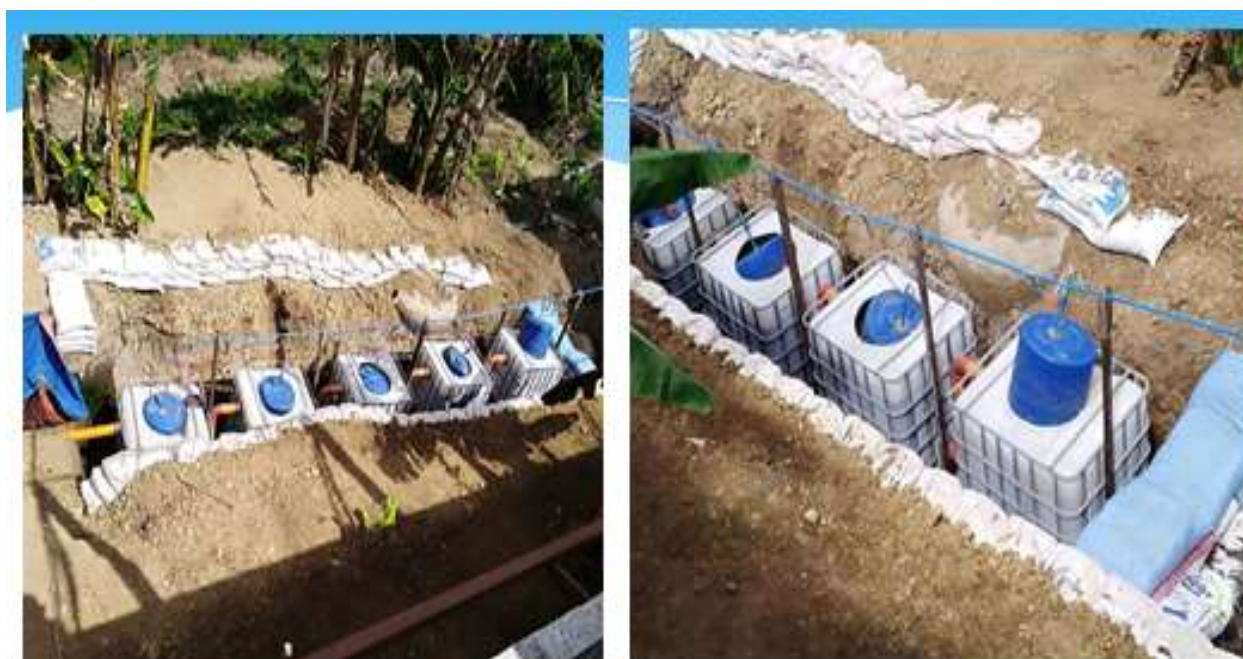
Ka Popoy Piggery located at Brgy. Litlit, Silang Cavite , Five (5) IBC Water Tank Biogas Digesters capable to treat 5 cubic meters volume of waste water.
