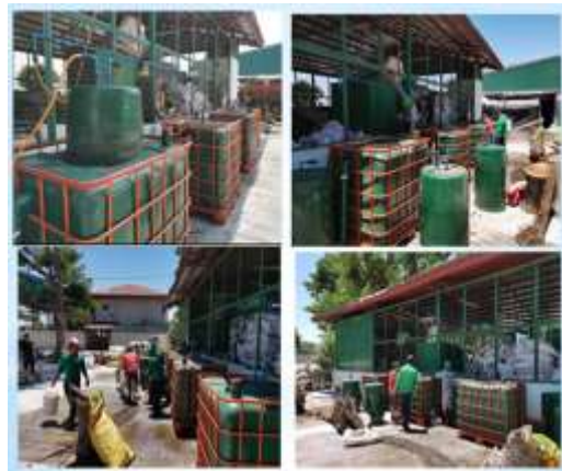
4 Cubic Meters IBC Water Tank Biogas Digesters of LGU Gen Trias.
