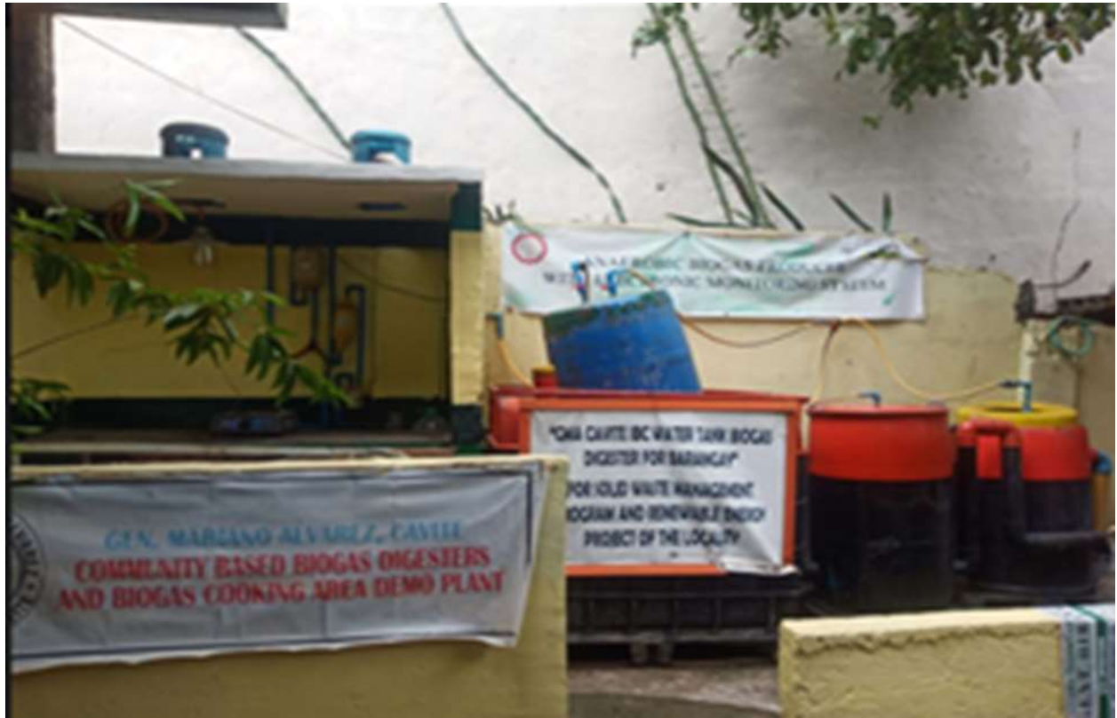
IBC Water Tank Biogas Digester with Communal Kitchen located at Brgy Poblacion 1, Municipal Compound, Municipality of General Mariano Alvarez, Cavite
