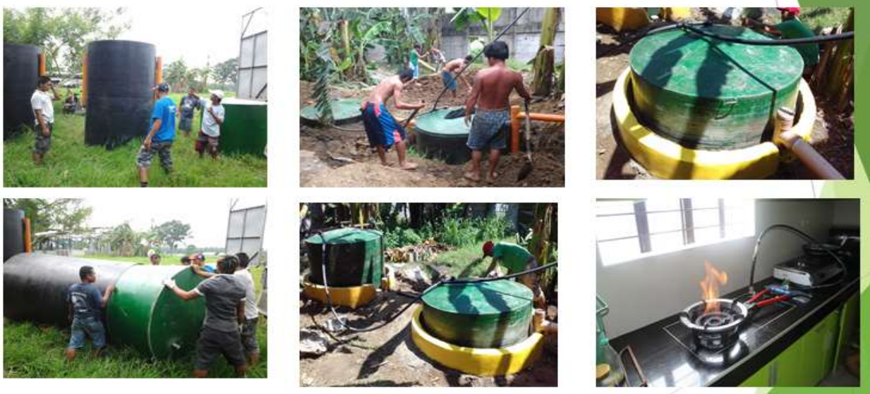
The actual installation of 60 Cu. Meter Two Floating Type Biogas Digesters at Sally Villapando Slaughterhouses located at Brgy. Poblacion 5, Gen. Mariano Alvarez, Cavite. (2017)
