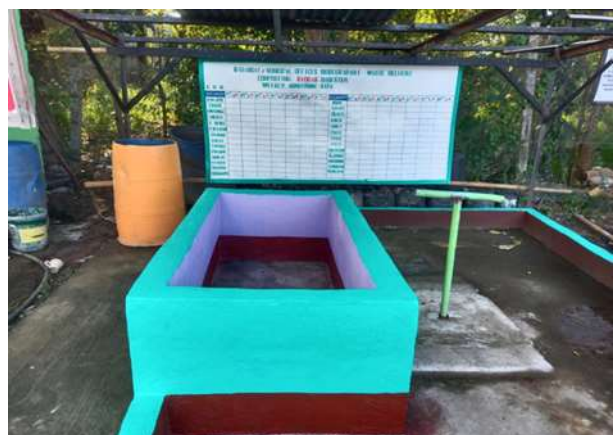
80 Cubic Meters (2 Tons) Capacity of Biogas Digester
